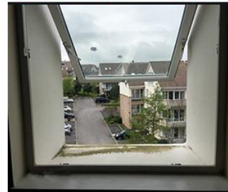
Without Window Restrictor-DANGER
